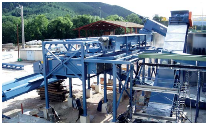
Installation with 3 x SH11-4
