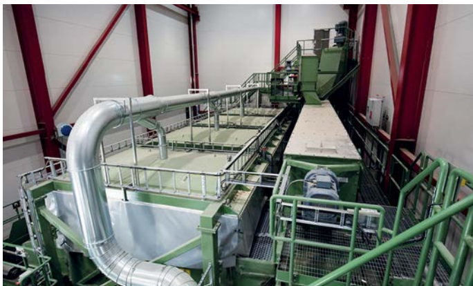
Installation with 4 x SH11-4
